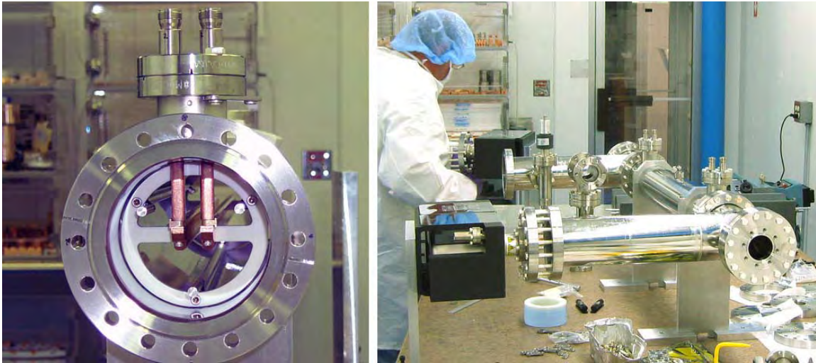
Figure 1. Kicker assembly. Left photo: electrodes, visible inside the vacuum vessel. Right photo: installing ion pumps.
