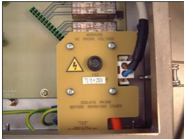
Figure 4: AC Mains Cover Board in Place
